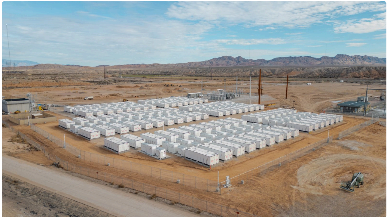
Figure 1. Battery energy storage at the Reid Gardner site, Nevada. Photo: Sig. Chiocciola / Wikimedia Commons (CC0).
